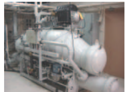
Water- and air-cooled chiller testing facilities
