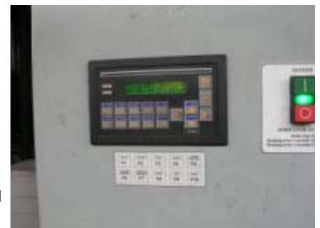
Chiller control panel
